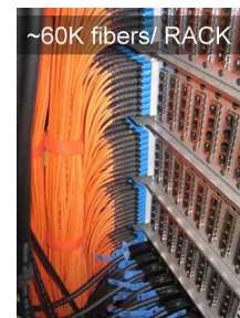
Fig. 10. Partially populated optics cables in an IBM Power 775 supercomputer rack.
